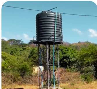
5,000-liter storage tank
