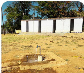
Hand wash tap stations installed outside bathrooms
